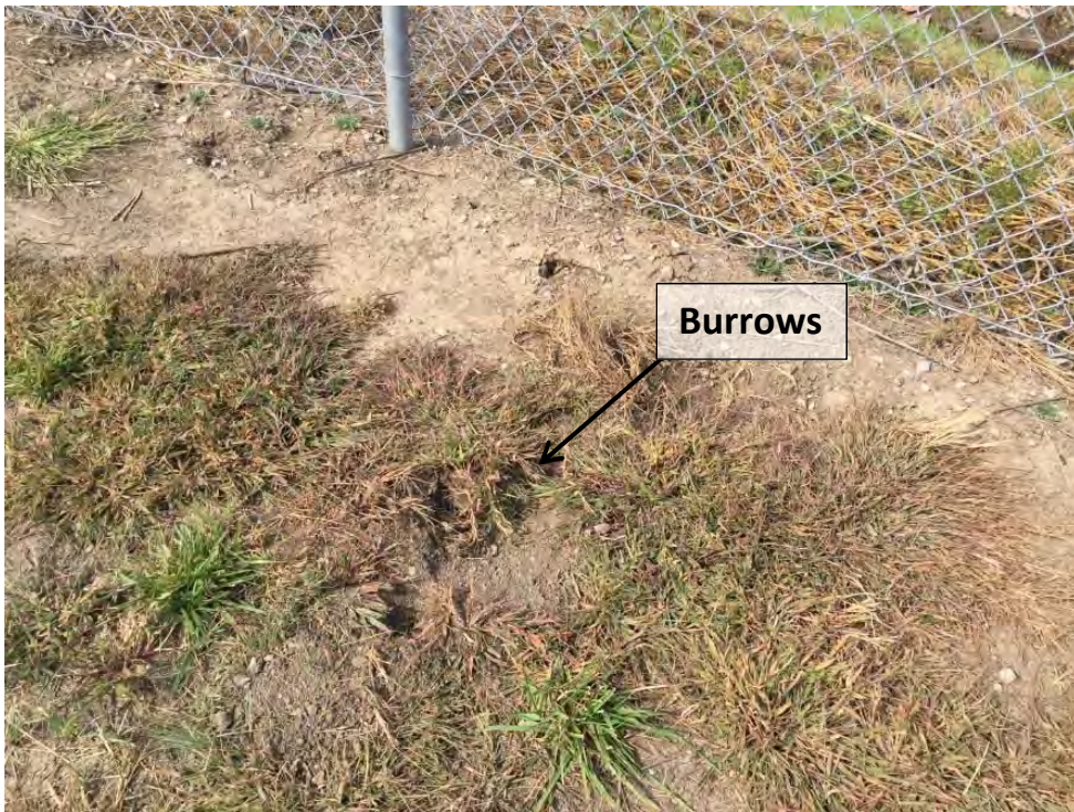
Photo No. 18 Burrows at Top of North Downstream Slope
