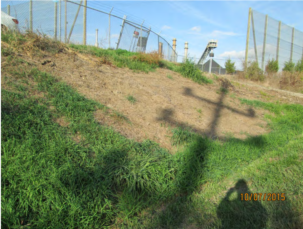
Photo No. 15 Dead Spots on South Downstream Slope
