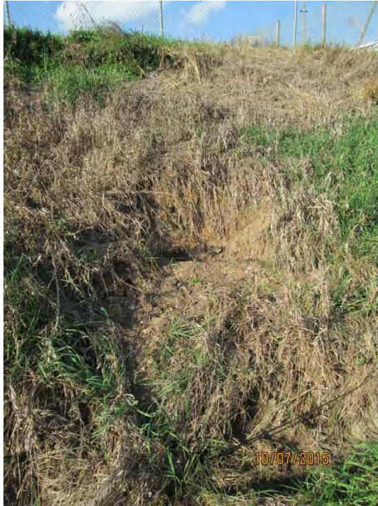
Photo No. 17 Slough on South Downstream Slope
