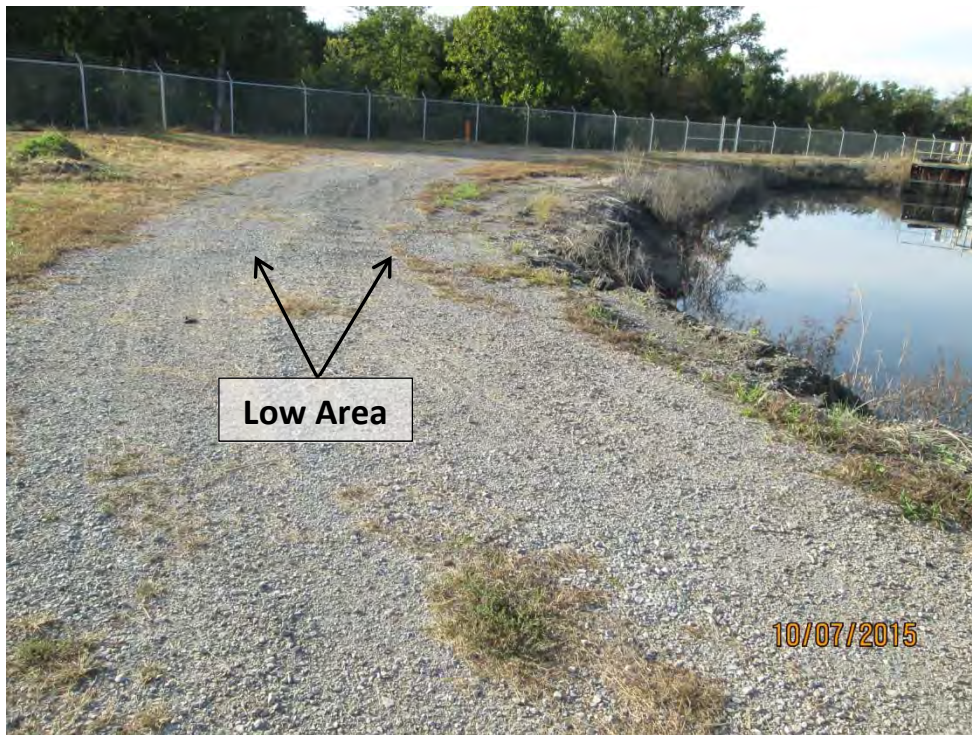
Photo No. 7 Low Area on South Crest
