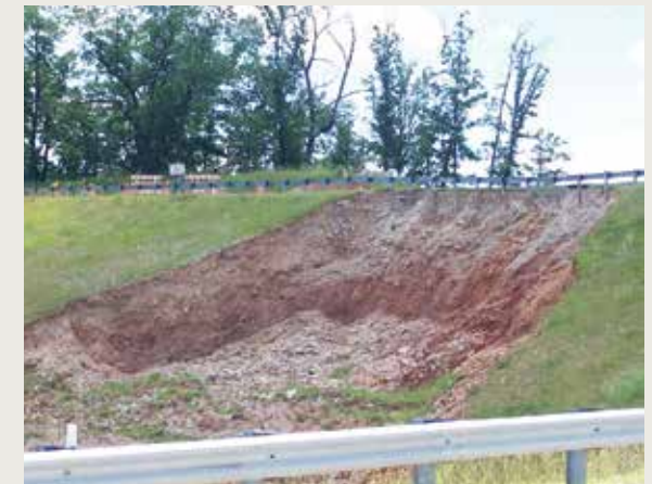
Landslide along a Missouri roadway.
